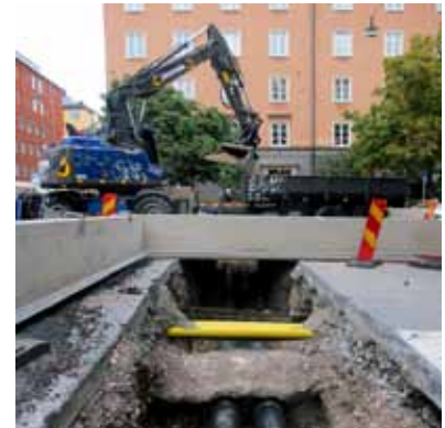
Modern insulated pipes make it possible to connect large areas to a common heat grid. Here a new pipe is laid in a street in Stockholm.
