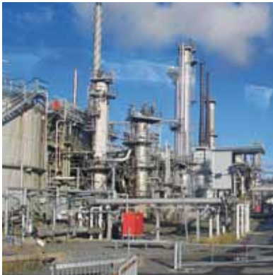
The production unit for tall oil diesel at the Preem refinery in Gothenburg.
